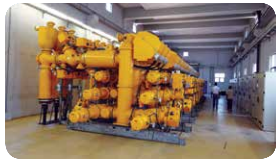
Kelanitissa Grid Substation, which will be augmented under this project
