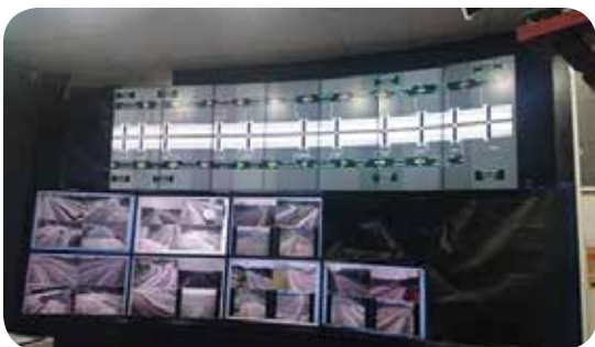
Displays at the control center
